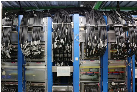
Cables carrying analogue signals from calorimeters.
